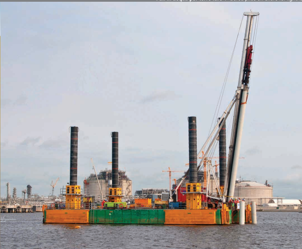
Pali in acqua per torre faro / Bored piles off shore for lighthouse
